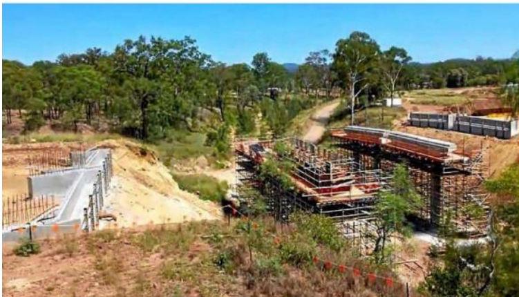
ONLINE VIDEO: The one-minute time-lapse clip from Nexus shows work being completed at the Rocky Gatton Creek bridge.
