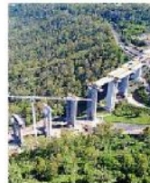
RANGE CROSSING: Oversized deliveries will be made to keep the project moving.
