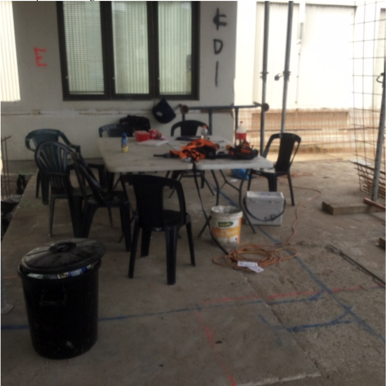
Non compliant Cribbing facilities - this is in the middle of the work site
