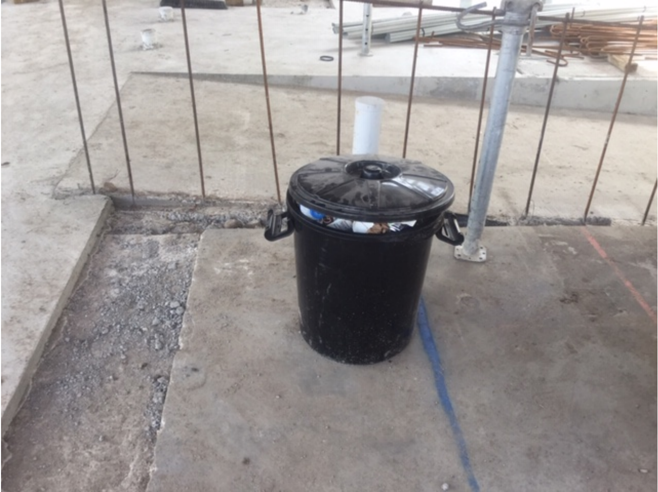
The Crib bin overflowing
