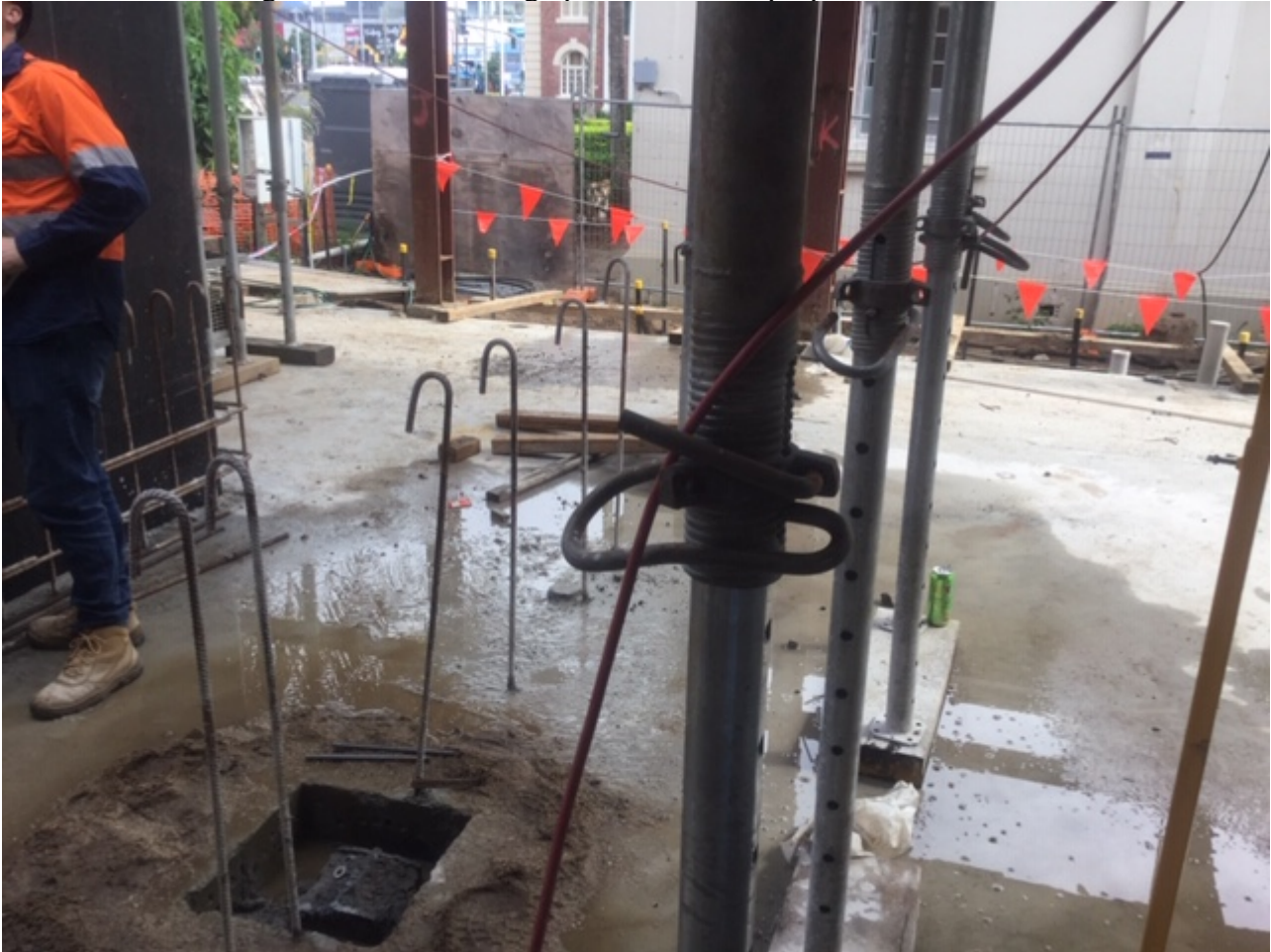
Protection of leads again - this time strung up on metal acro props
