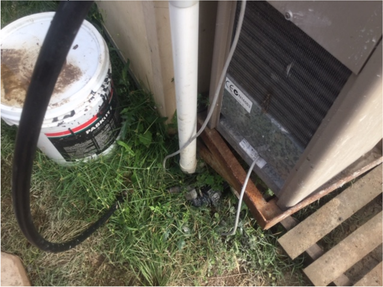
Another lead not protected
