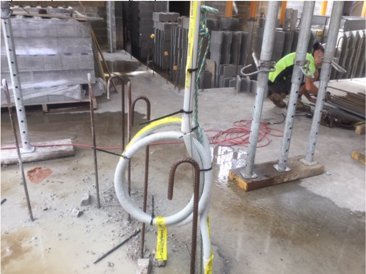
Exposed Temp Construction Wiring / not protected
