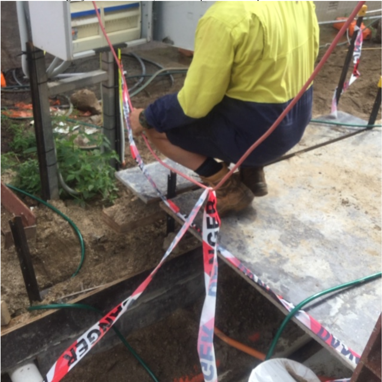
A worker working adjacent to a fall risk, over a star picket with no protection
