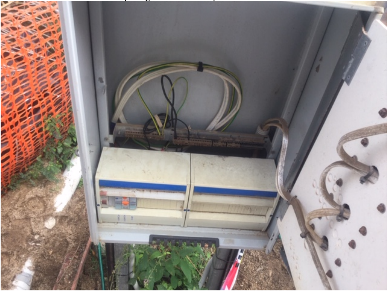
Switchboard Patel not secure exposing workers to live parts
