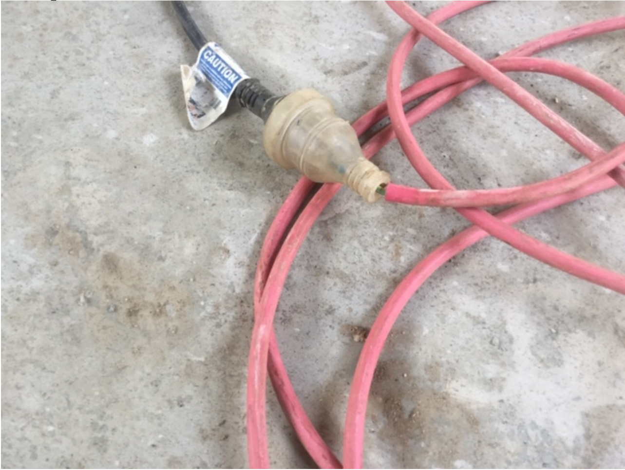
A damaged extension lead
