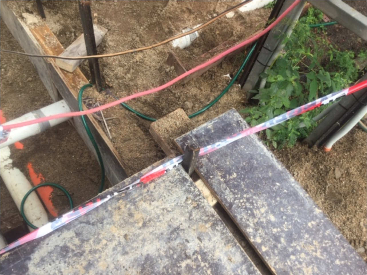
These photos are from the switchboard access platform
