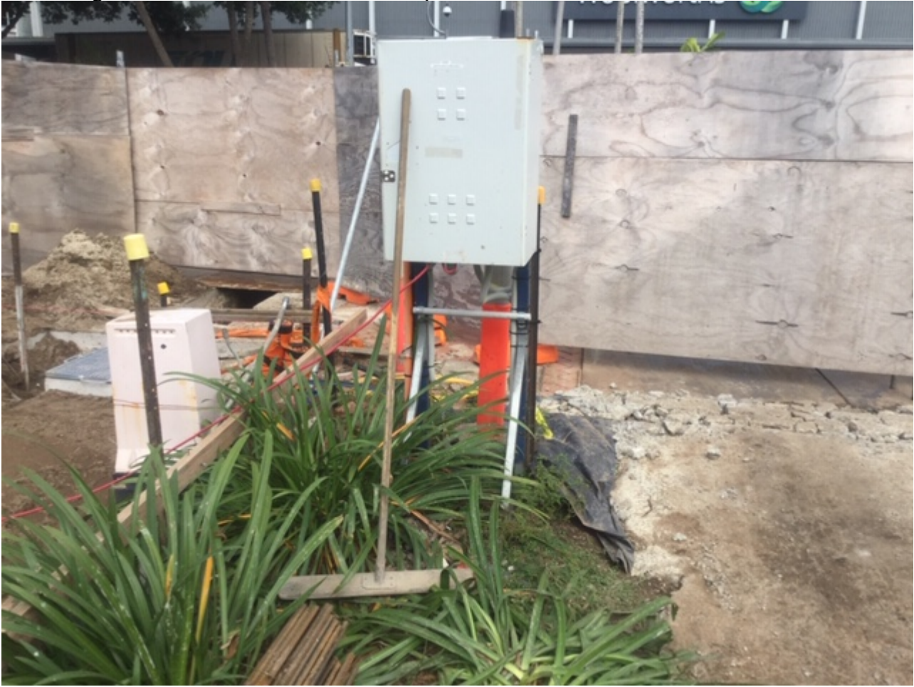
Not having Access of 600mm unincumbered space around a switchboard
