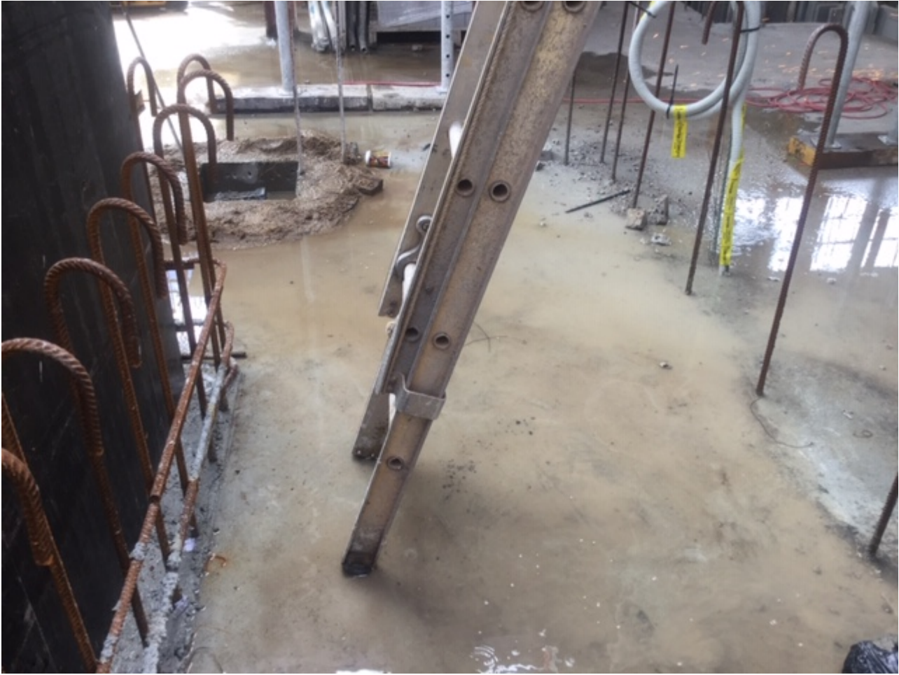
Ladder not secured
