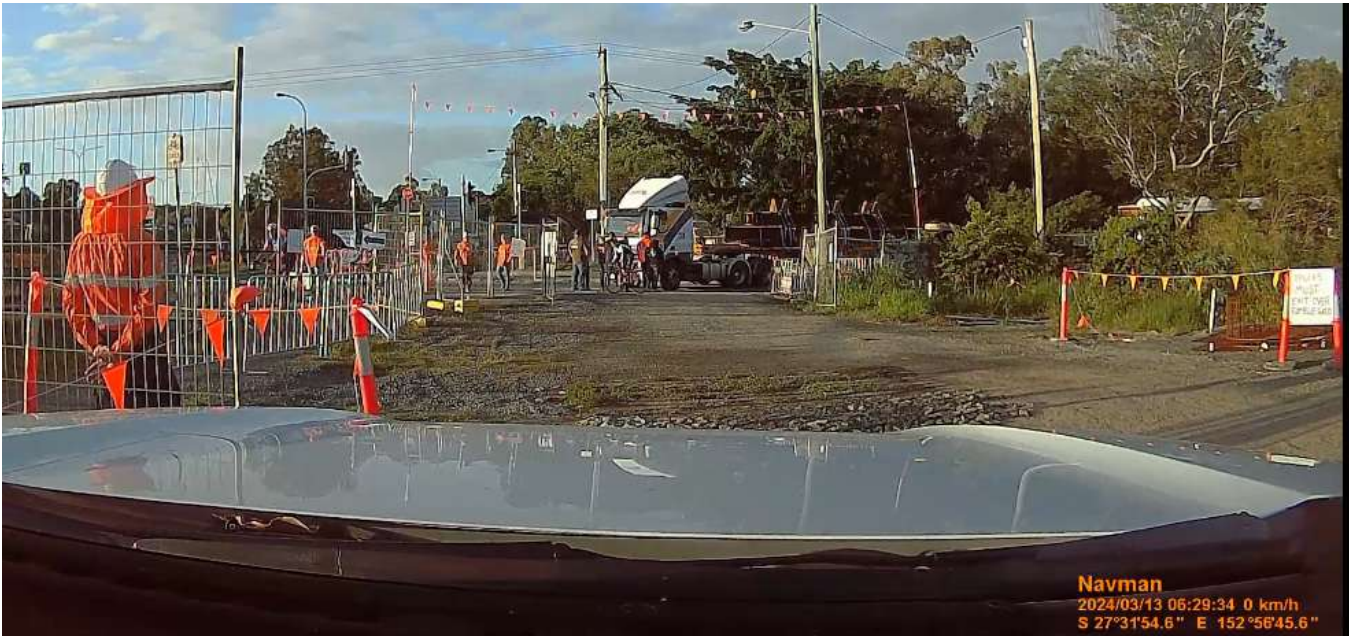
6:35am Police on-site
