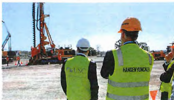
Piling work starts at on USC Moreton Bay's foundation building. Source: Pine Rivers Press.
