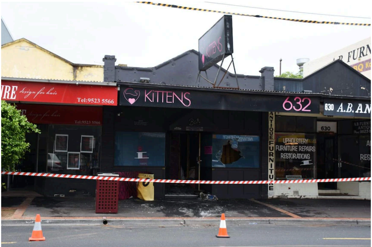
The fire gutted the Kittens strip club and caused significant damage. (ABC News: Margaret Paul)
