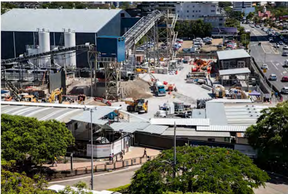
Construction work on the Cross River Rail Gabba station in January. ATTILA CSASZAR
