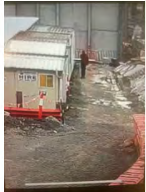
Dutton Park Station, 3 May 2024: masked intruder accessed site from 6:15am for approx. 10 minutes and took photos. Concerns of sabotage.
