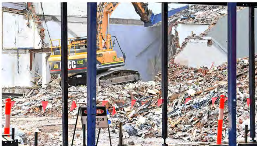
Construction work at the corner of Mary and Albert st, Brisbane. Wednesday November 4, 2019. (AAP Image, John Gass)
