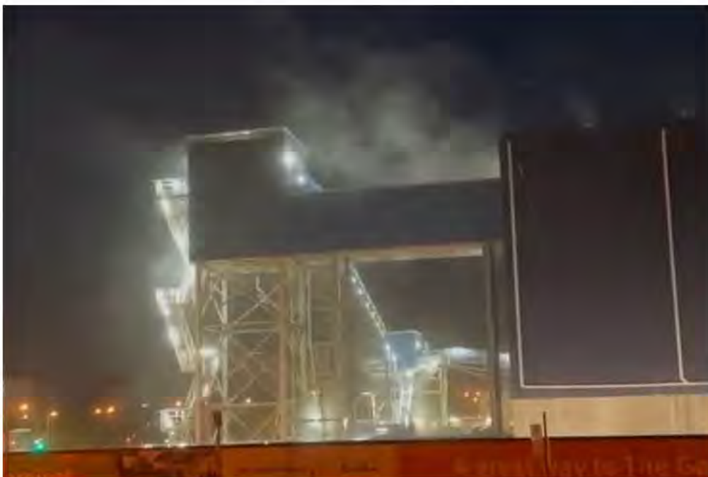
Dust being released into the air from the Woolloongabba Cross River Rail worksite.
