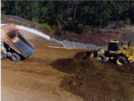
Tonka trucks are being used on the Toowoomba Second Range Crossing project. contributed THE Toowoomba Second Range is showcasing some of road building's biggest machinery.
